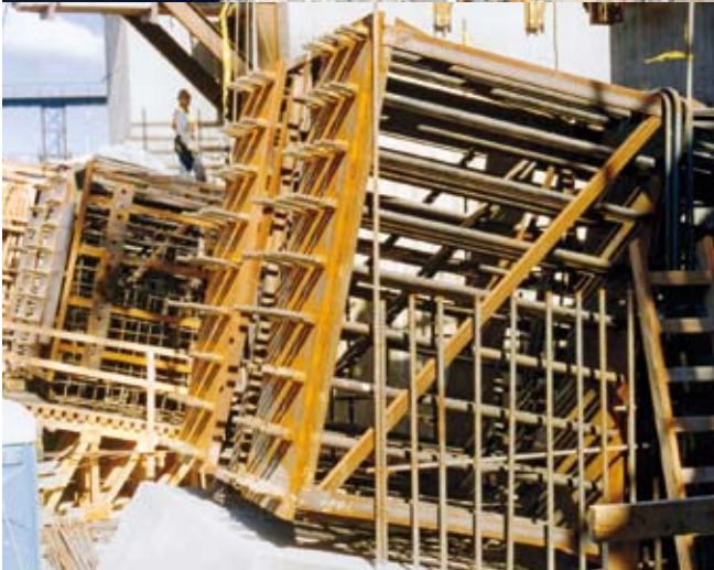
Grand-Mère Generating Station, Canada
